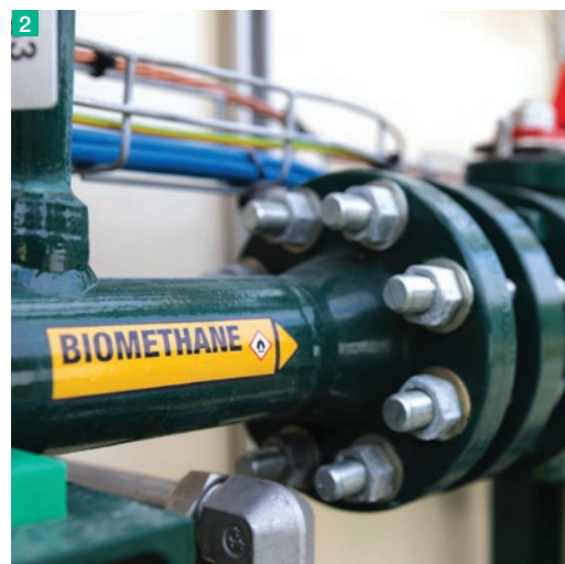
1 Anaerobic digestion plant
